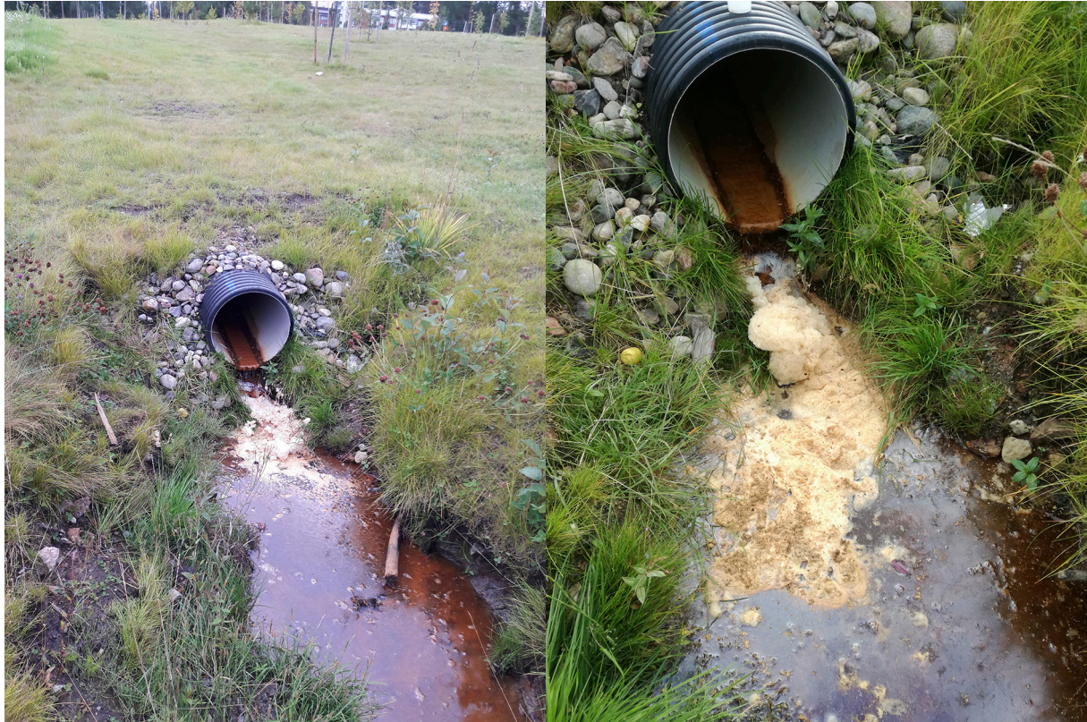
Figure 20a and b Contaminated run-off water outlet.
