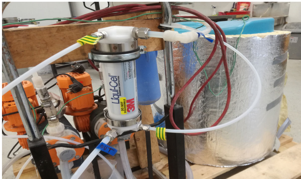
Figure 18 Liqui-Cel membrane unit, heater of inlet water, and a pumping station.
