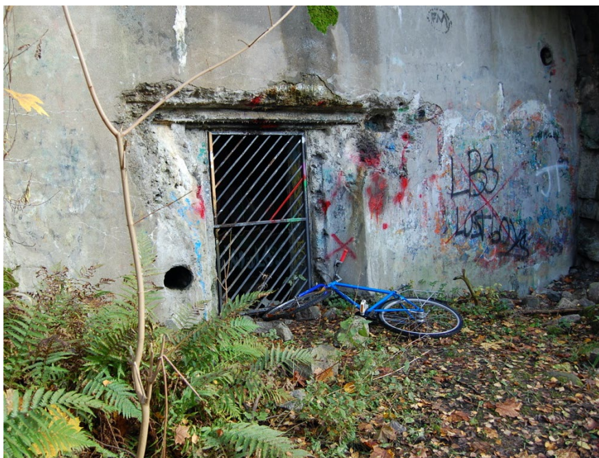
FIGURE 30 Picture of the entrance of the First World War bunker at Vartiokylä Hill Fort in 2012. Photo: Heidi Wirilander 2012.
