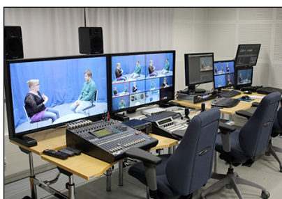
Figure 3: The control room
