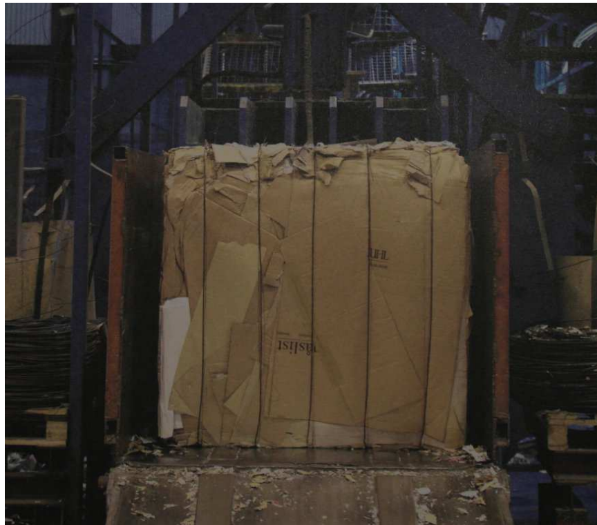
Figure 2. Baling machine in use at Gufunes Baling & sorting plant (SORPA 2013a).
