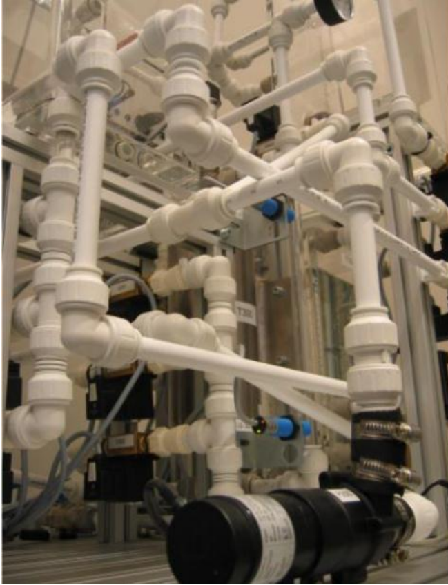
FIGURE 12 Heat production plant
