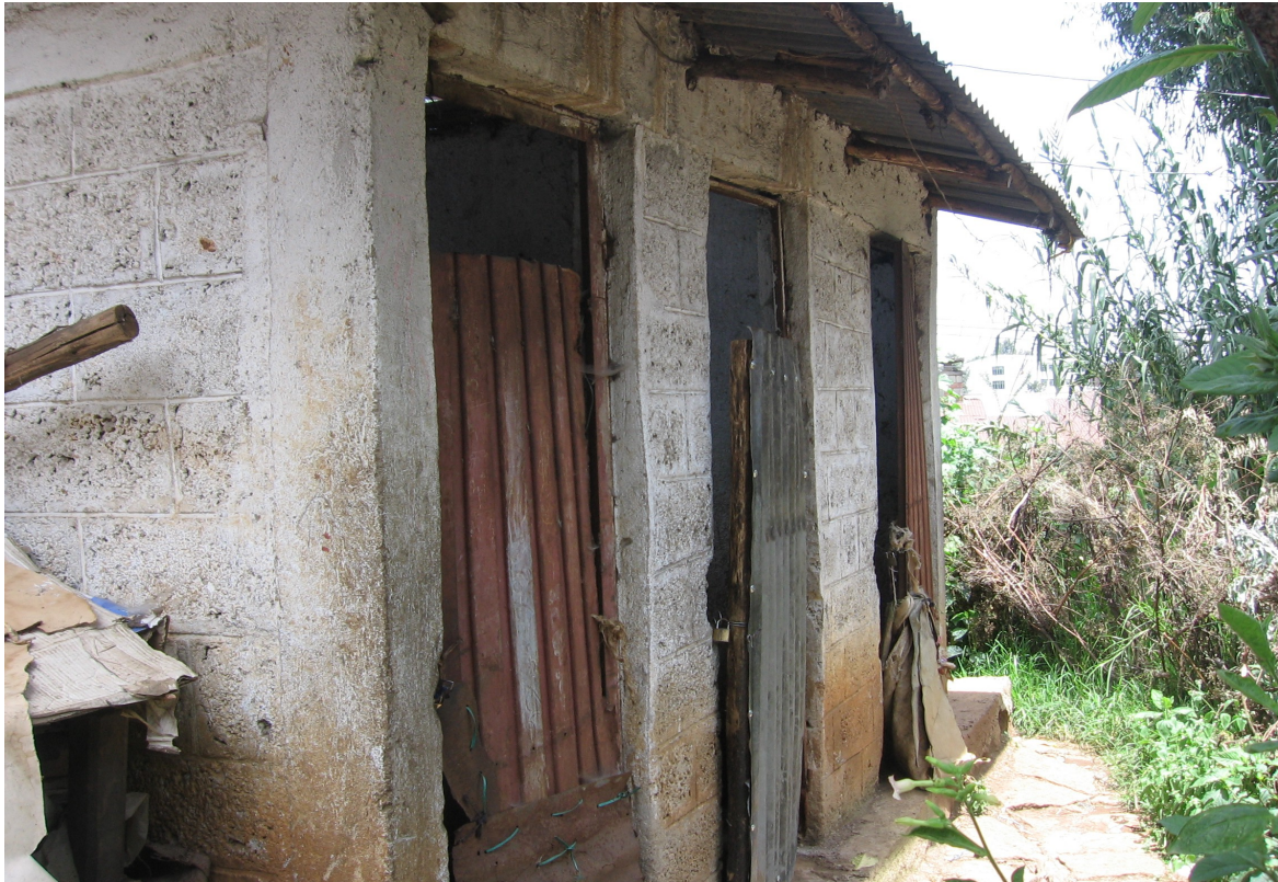
Photo 6: Three toilets of the compound of Yeiyeneabeba (Photo: Maija Suomela)
