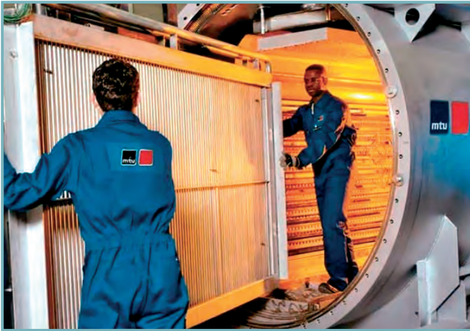
FIGURE 18. Installation of a fuel cell stack at a MTU CFC plant in Germany. Photo: www.mtu-online.com
