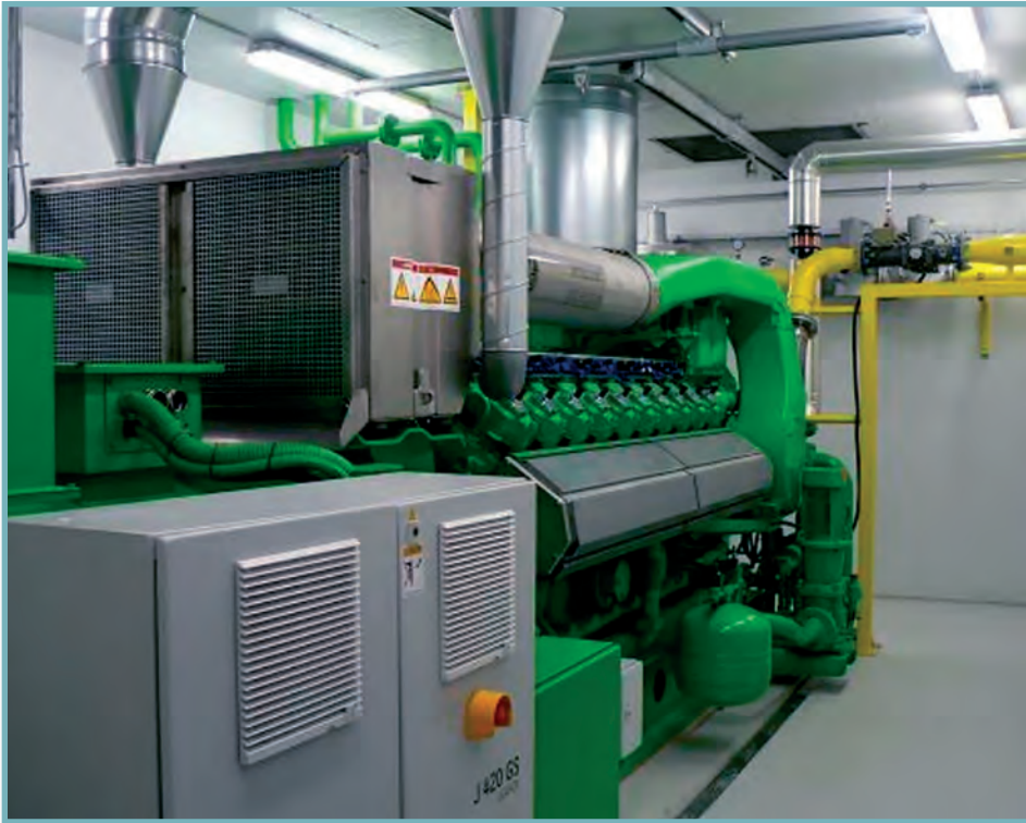
FIGURE 17. IC gas engine (piston engines). Example of a piston engine in a CHP unit, a 20-cylinder Jenbacher gas engine. Photo: ge-energy.com (Jenbacher)
