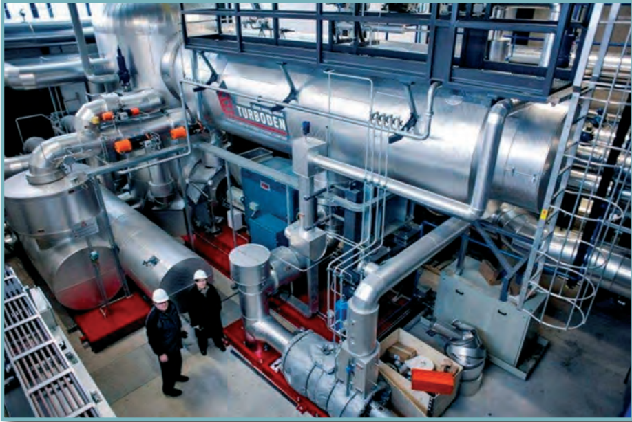
FIGURE 14. Turboden ORC plants are factory installed on the platforms, and during the assembly in the CHP plant they are connected together and to the boiler. The ORC-CHP plant in the picture is in Toholampi, Finland, and the power output is 1.3 MWe. Photo: Turboden.it
