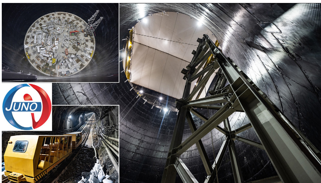
↑ Figure 1. JUNO construction status. View from the bottom (big photo) and from the top (upper inset) of the water pool. Lower inset: cable car at the end of the slope tunnel.
