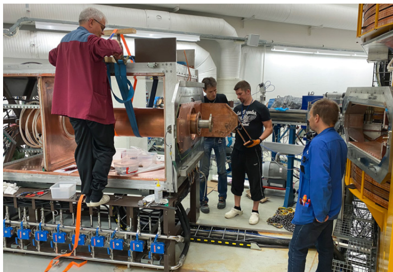
← Figure 1. Photo of technical team working on refurbishing one of the K130 RF cabinets.
