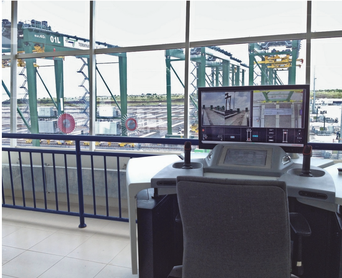
FIGURE 5 One of the remote operator stations installed in the Lamong Bay Terminal with the main display showing some of the final UI design solutions © Konecranes
