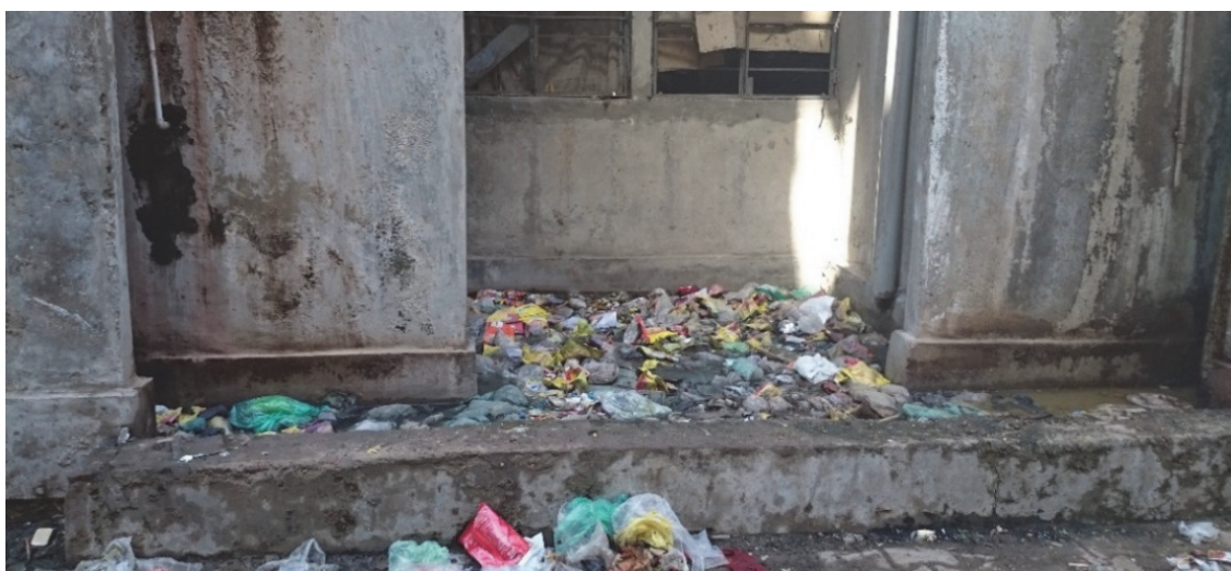
FIGURE 6.8. A wall meant to block flooding on the street, February 2016.
