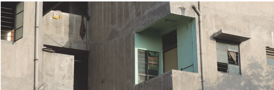
FIGURE 6.1. Many windowpanes have fallen down from the buildings, May 2015.
