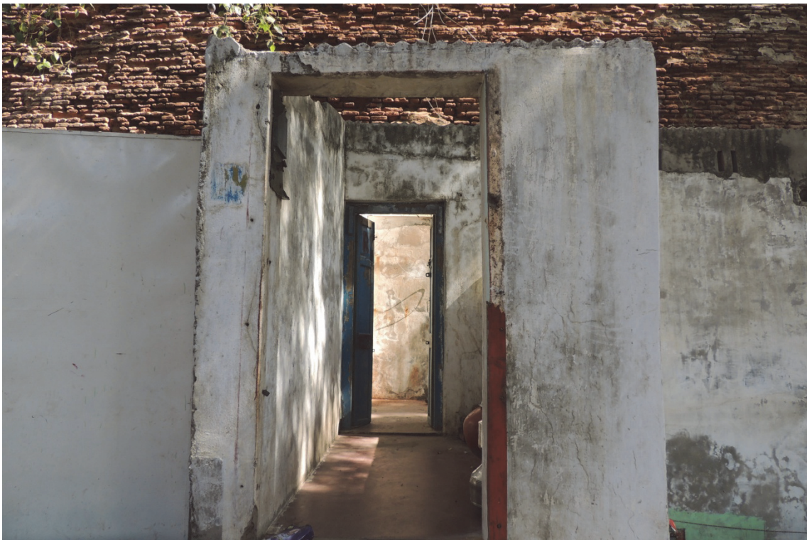
FIGURE 4.1. Remains of demolished houses at the riverfront, January 2016.
