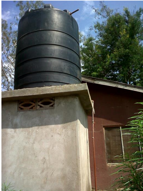
Plate 12: Water tank (5000L) connected to the WP700 Source: MWAKANGALE (Nov. 2014)
