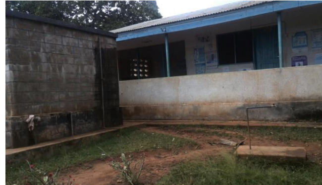
Plate 2: A water tank and a tap (Water is used for washing and cleaning purposes at the dispensary) Source: MWAKANGALE (Sept. 2014)
