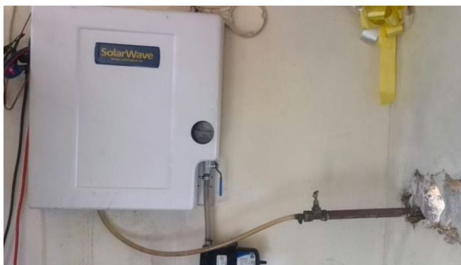
Plate 5: Connection of the water purification unit in the store Source: MWAKANGALE (Sept. 2014)
