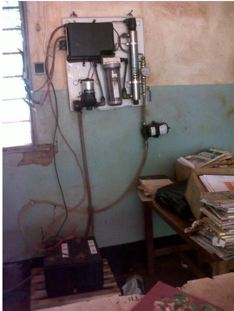
Plate 8: Connection of the Purification System WP700 at Teachers' Office Source: MWAKANGALE (Nov. 2014)
