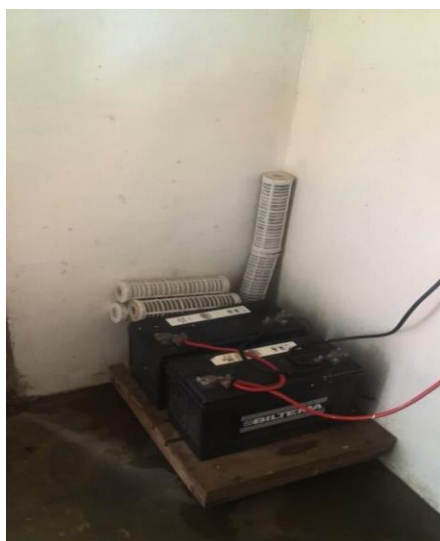
Plate 7: A battery to run the installed system (WP700) Source: MWAKANGALE (Sept. 2014)
