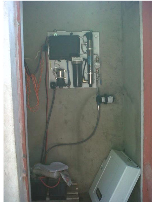
Plate 13: Connection of water purification unit in the store Source: MWAKANGALE (Nov. 2014)
