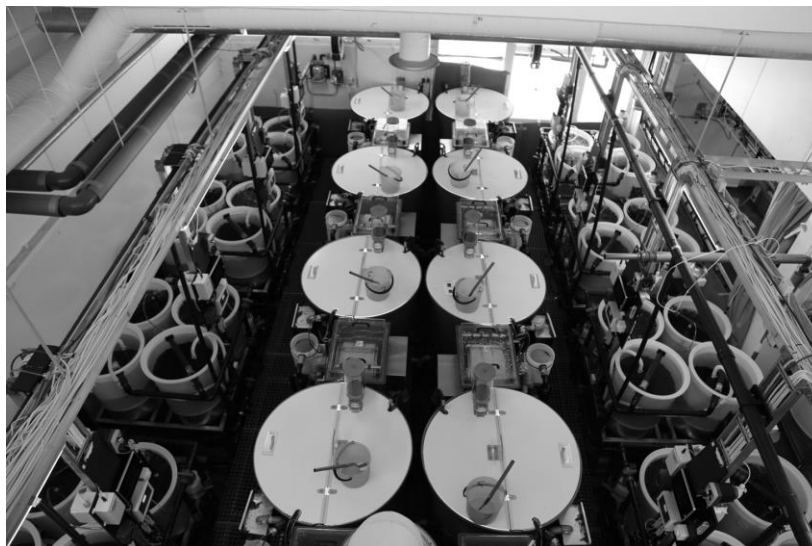
Figure 2. Laukaa Fish Farm Experimental RAS Facilities
