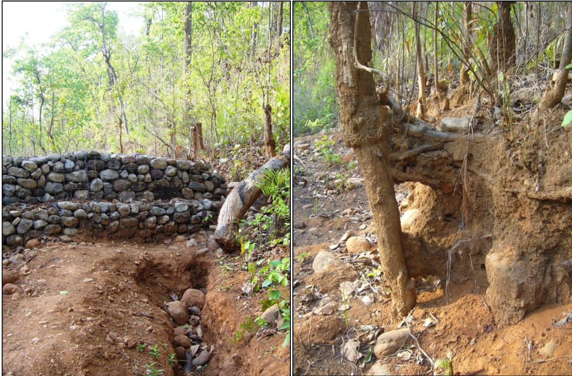
Figure 7. On the left: Dam structure constructed using gabion box to protect sedimentation tank of Nayabelhani scheme has been damaged several times during floods. On the right: Impacts of soil erosion caused by flooding visible near the water source of Nayabelhani scheme.
