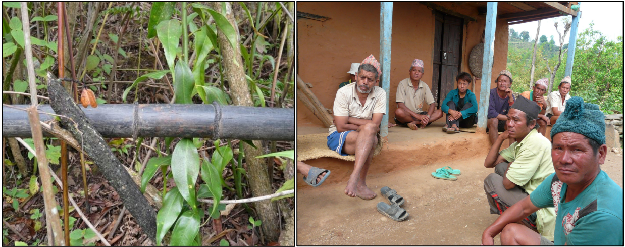
Figure 12. On the left: Leaking pipe from Ruchang A scheme repaired using old leftover pipes from the construction time. On the right: Water users and users committee members of Ruchang C scheme during the focus group interview.
