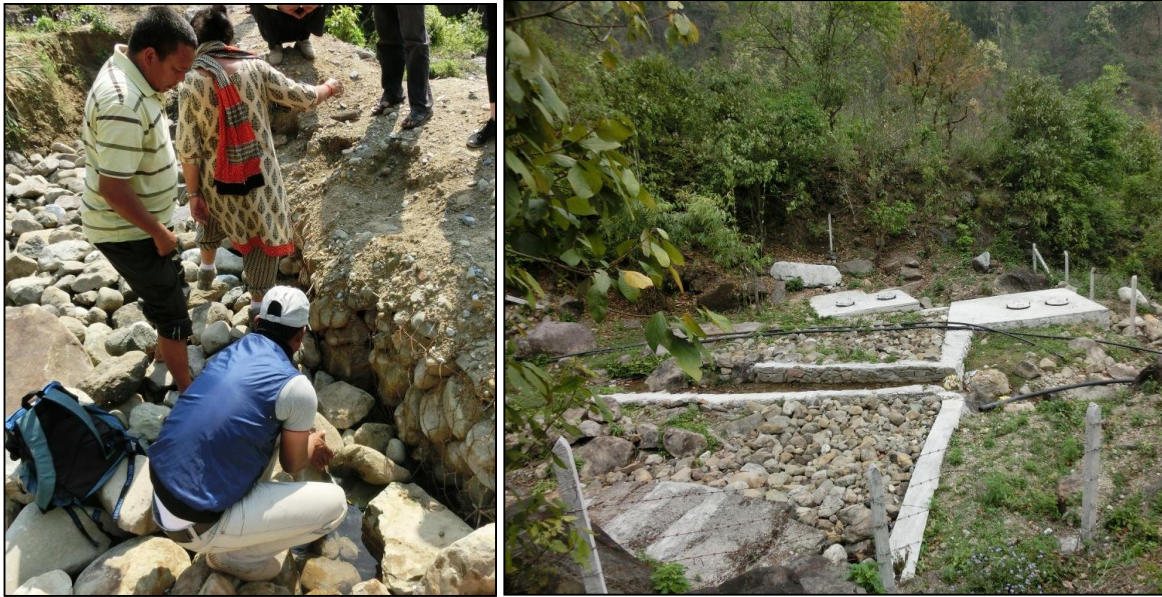
Figure 10. On the left: Gabion box used at the water source area of Rambas Sitabas and Aaptari schemes to protect water intake from flooding. On the right: Fenced source area of Rambas Sitabas and Aaptari schemes with collection chambers.
