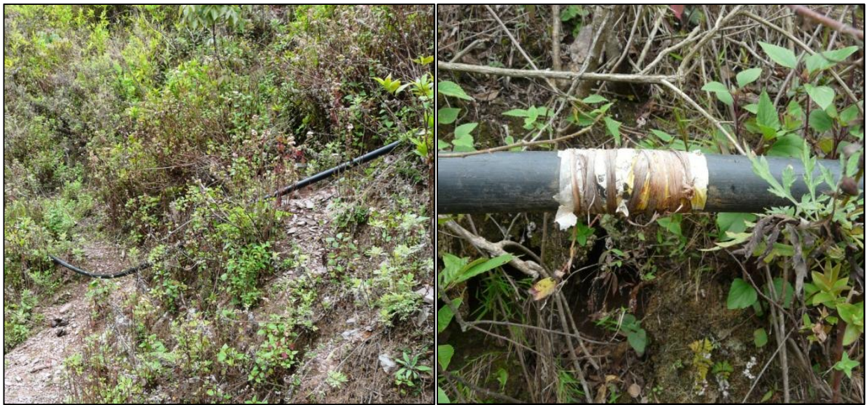
Figure 6. Uncovered water distribution pipes along the hill slopes in Ruchang village. Damaged pipe repaired using a piece of plastic.
