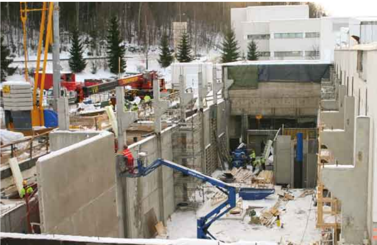
Fig. 1. The construction of the Accelerator Laboratory extension, which will house the new MCC30/15 cyclotron and the IGISOL facility.
