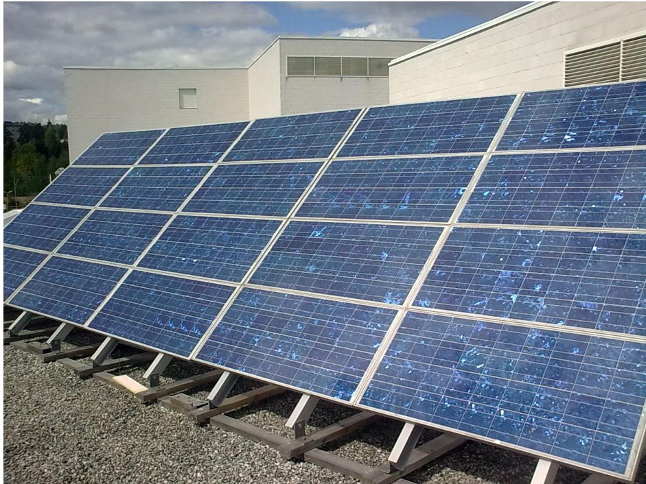
Figure 7: A photograph of the Agora polycrystalline PV system.
