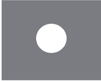
FIGURE 57 A clear hole in the wall.
