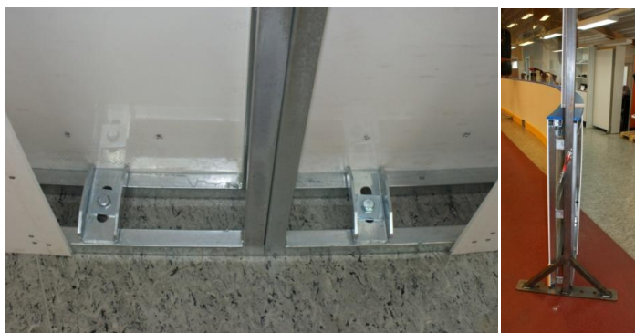
FIGURE 12. Anchoring system (left) and special posts located at both ends of the dasher board to support it (right). (Photographs by Tuomo Hyvärinen)
