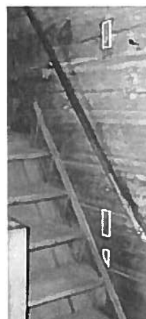
Figure 2. Three notches in the northern wall of the eastern cross-arm.
