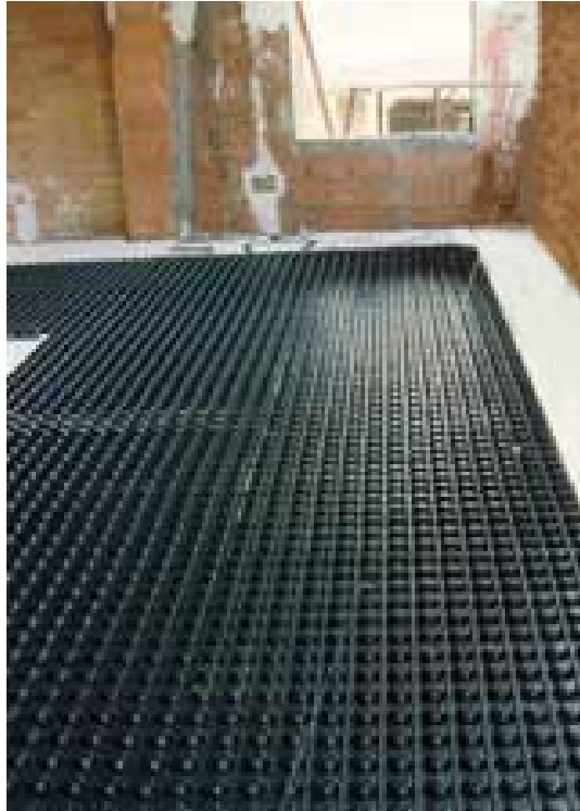
Figure 3.16. A photo of the PCM panels taken before laying the water pipes between the columns of PCM cone-frustums. This PCM assisted under-floor electrical heating system is produced by NetGreen Solar Ltd [77].
