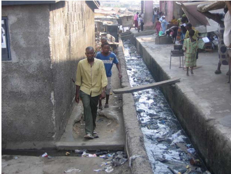
FIGURE 5 A typical state of sewage system in Lagos (Bidemi Coker)
