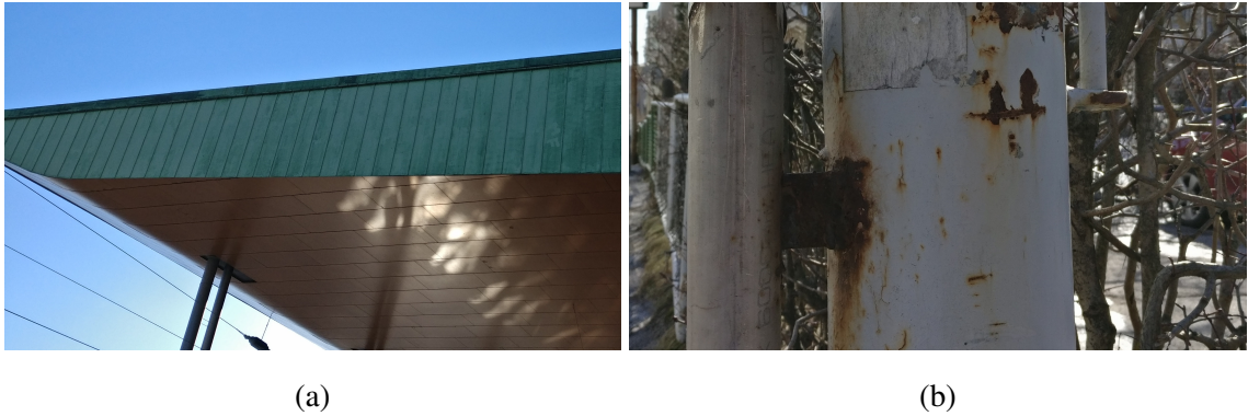
Figure 2: Figure (a) shows protective corrosion on a building facade. Figure (b) shows destructive corrosion on a gate pole.
