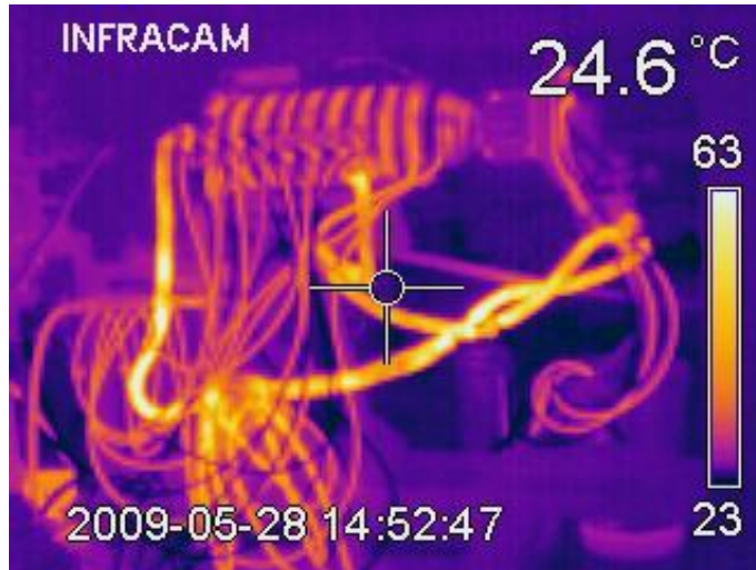
Figure 3.10: Thermal image of SAGE with 600 A of current applied on the coils. The hottest parts are the current carrying cables, at a temperature of approximately 60°C. The current carrying cables shown in this image were later changed to thicker ones lowering the cable temperatures close to 30°C.
