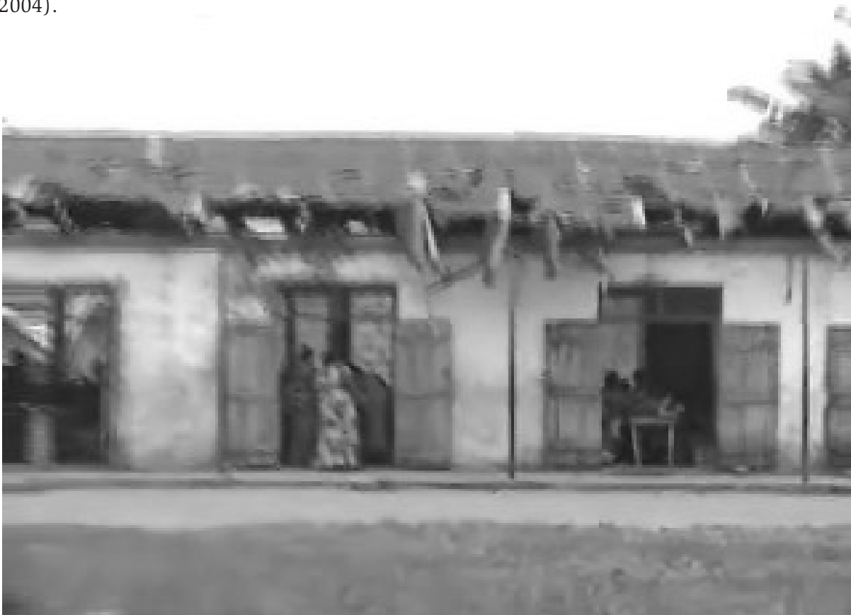
A dilapidated Primary school
