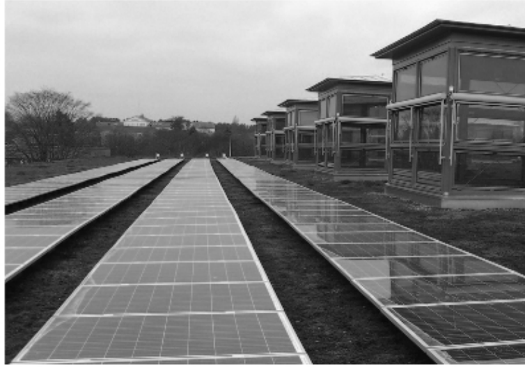
Figure 11: Example of an solar array installed on a horizontal plane. Linköping's public library in Sweden [Appendix 2].
