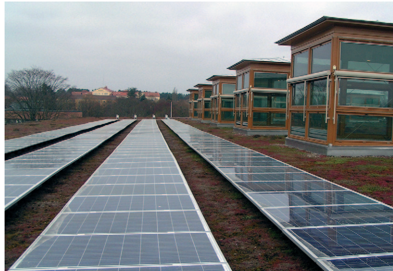
SwedModule's on Linköping's public library. The system is installed by Switchpower.
