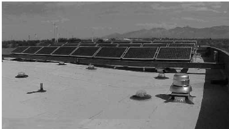
Figure 10: Example of row installed solar array [16]
