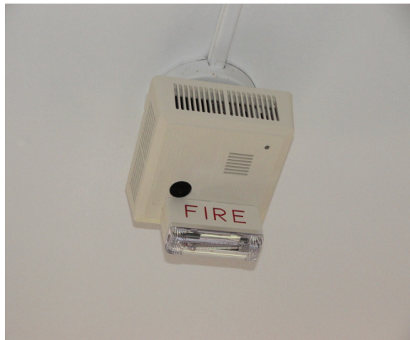
FIGURE 2. Audio/Visual Fire Alarm incorporating strobe light and buzzer.
