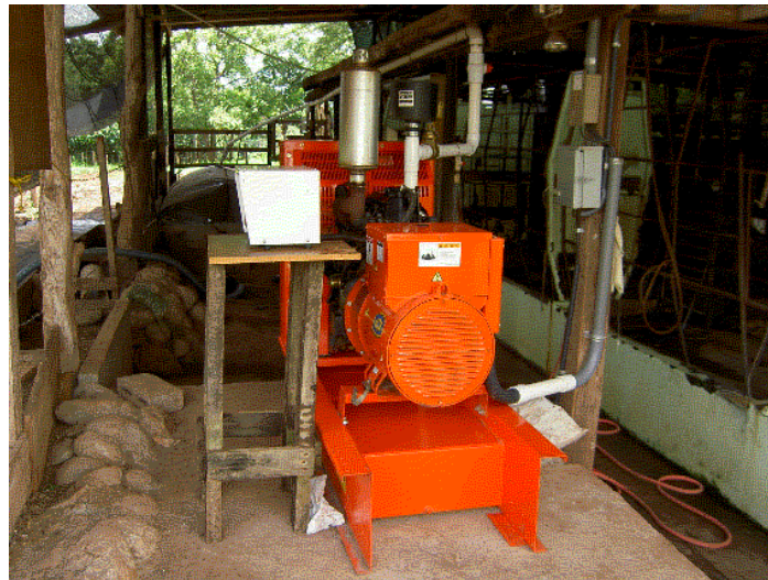
Figure 2. Dual-fuel Diesel engine for electricity generation.
